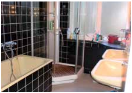
BEFORE: THE BATHROOM FROM THE 60S HAD ITS CHARM BUT WAS ALSO DARK, CRAMPED, AND IMPRACTICAL.
